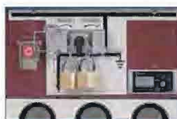
Earthed and locked position.
